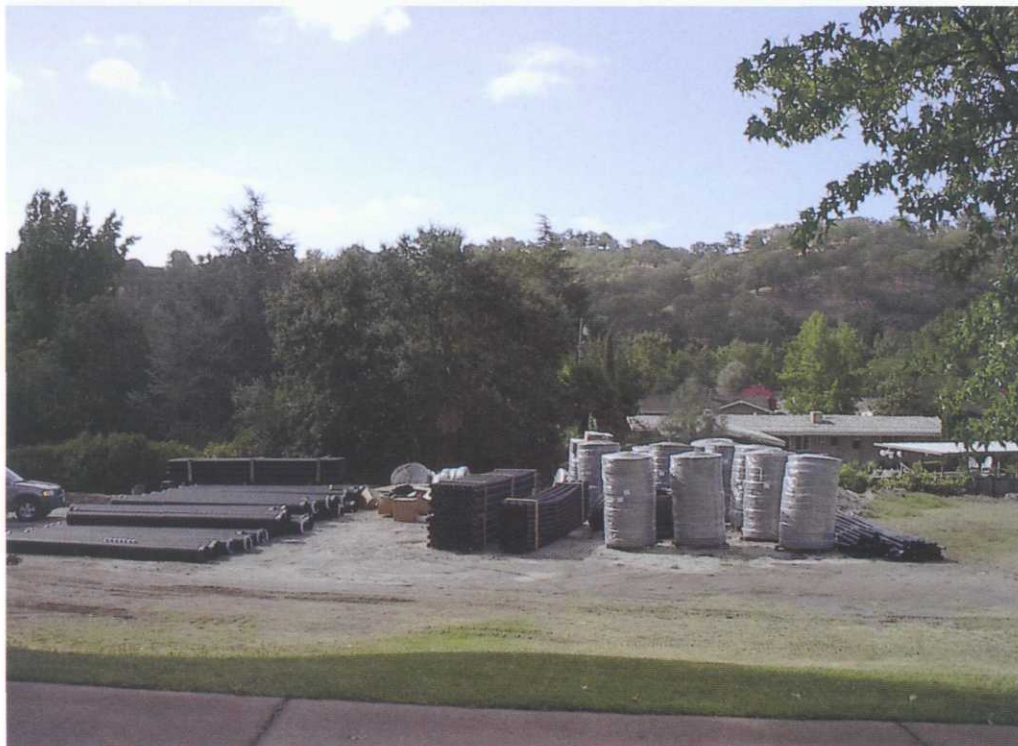
A large staging area allows storage of the new materials for a drainage project.
