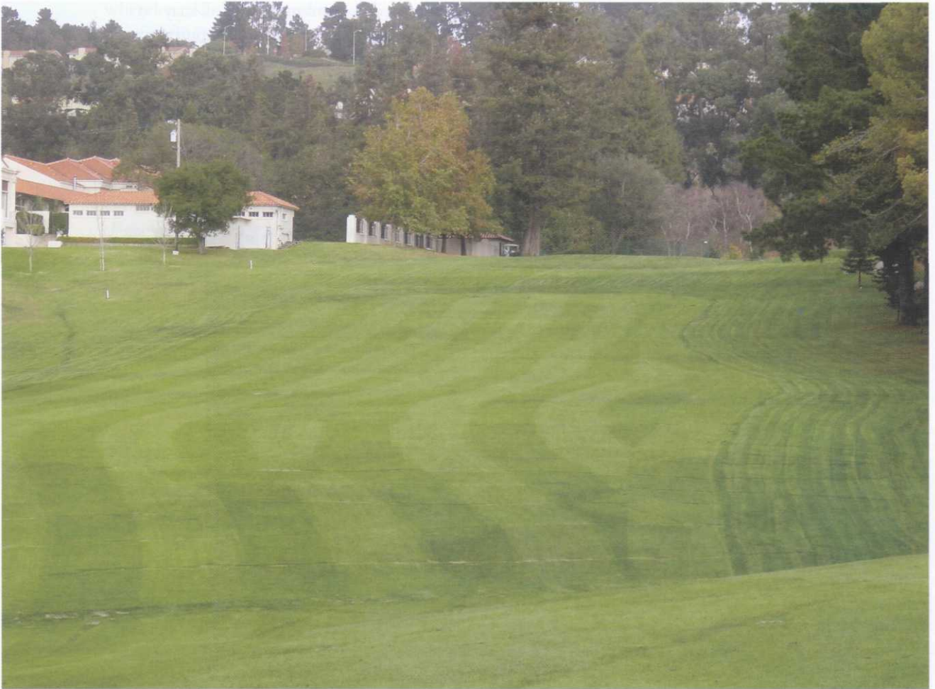
Sod lines over the new fairway drainage are almost completely healed only three weeks after the installation.
