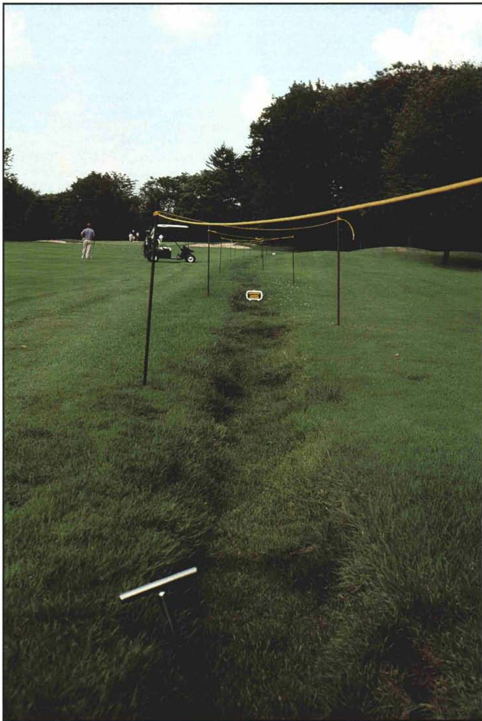
Sloppy construction — even the best contractor can have a bad day!
